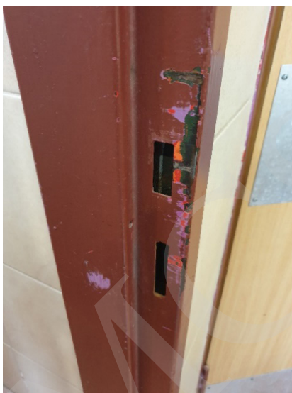
Figure 5. Peeling paint in the boys' bathroom – a photo taken by an activist and submitted as part of the retrial
